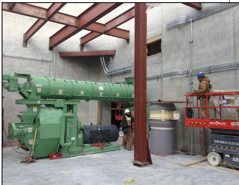
Interior of pellet tower
